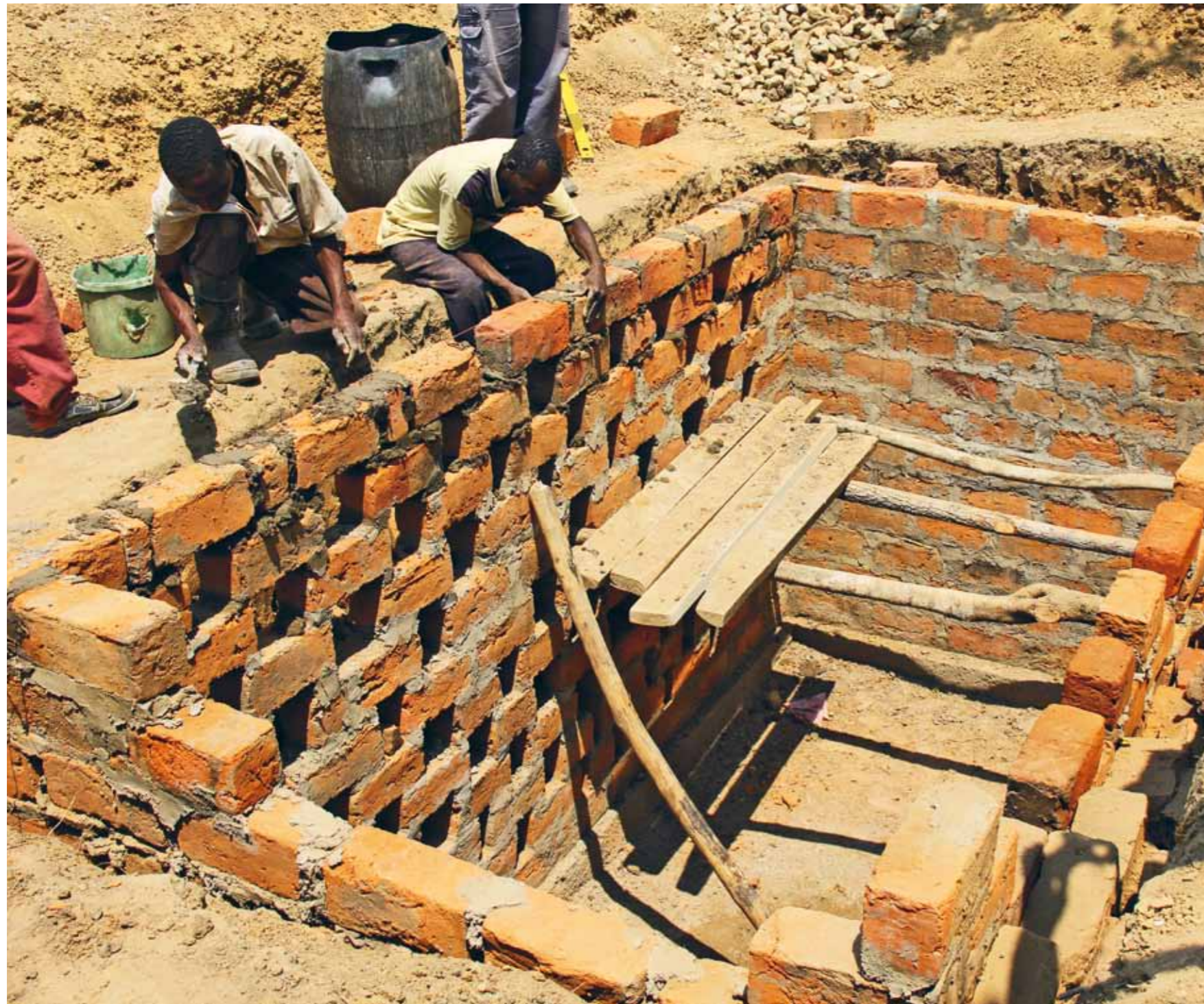
Sanitary construction by the community for Kabulembe School in Namayani, Chibombo District.
